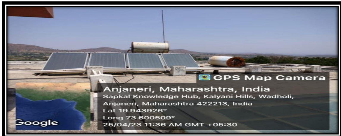
Solar water heater
