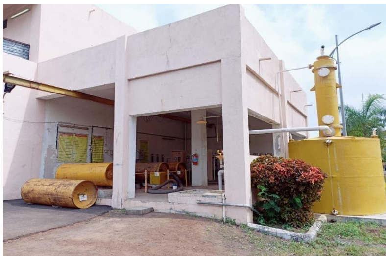
Photo: Chlorine Tank
