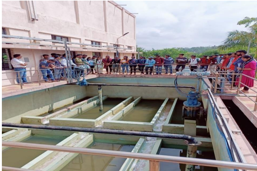
Photo: Rapid Sand Filter Bed
