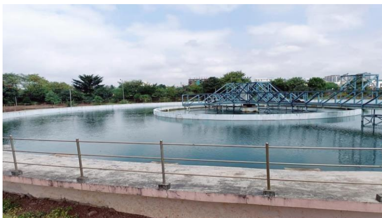
Photo: Sedimentation Basins
