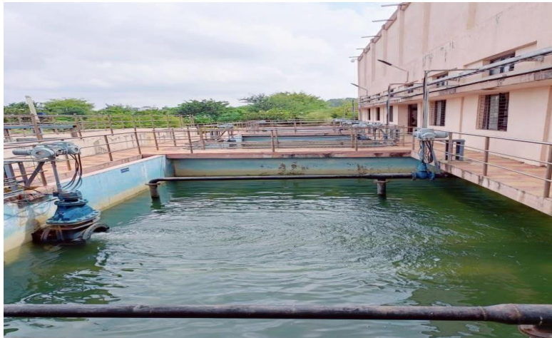
Photo: Flocculation Basins
