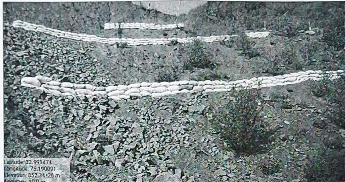
Sand bags at Co. 70/Udh. Morh Slip
