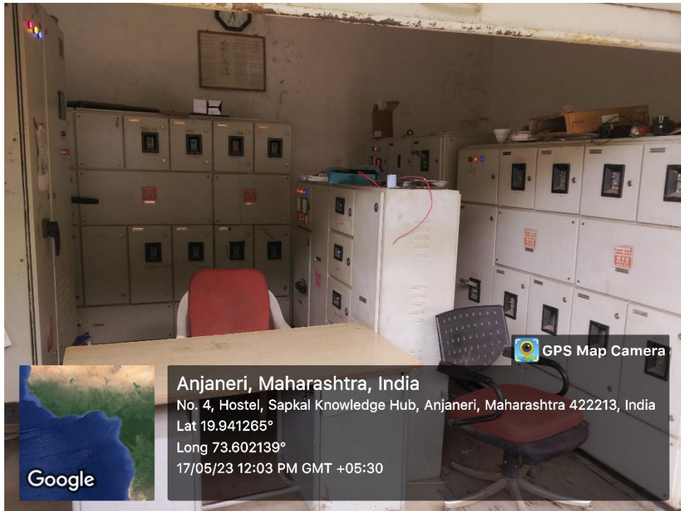
Geotagged Photo of Capacitor bank installed in campus
