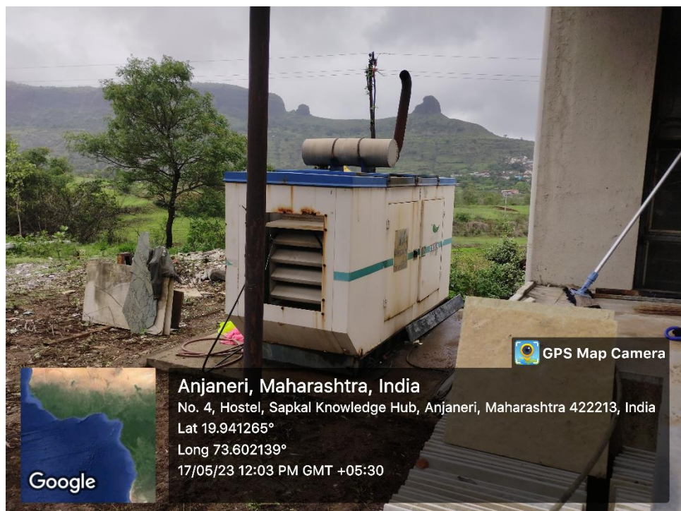
Geotagged Photo of DG Set installed in campus
