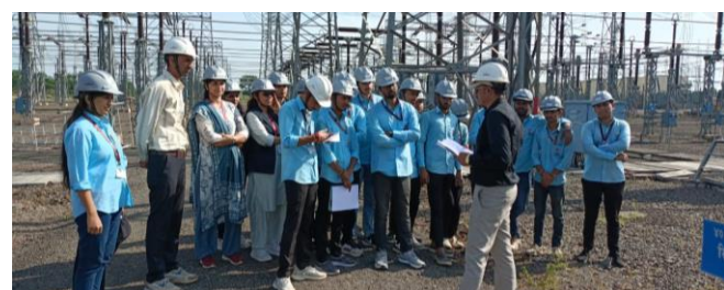
Visit at 400KV Substation Babhaleshwar, Dist. Ahilyanagar on 13 October 2025
